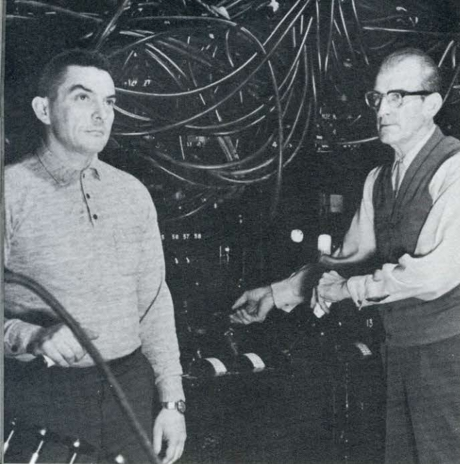
Electricians check equipment before start of TV show.
